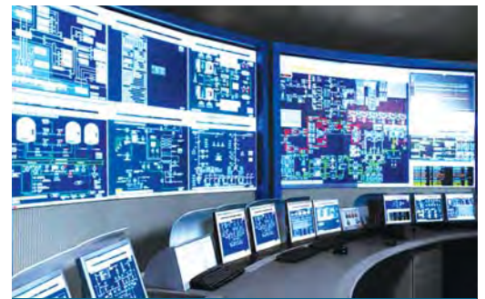
Data Management & SCADA
